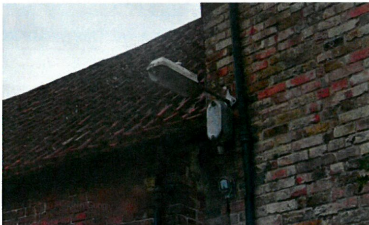
Bowling Street Light (before LED upgrade):
