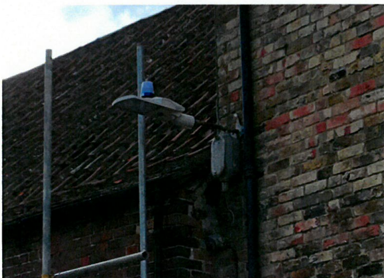
Bowling Street Light (after LED upgrade):
