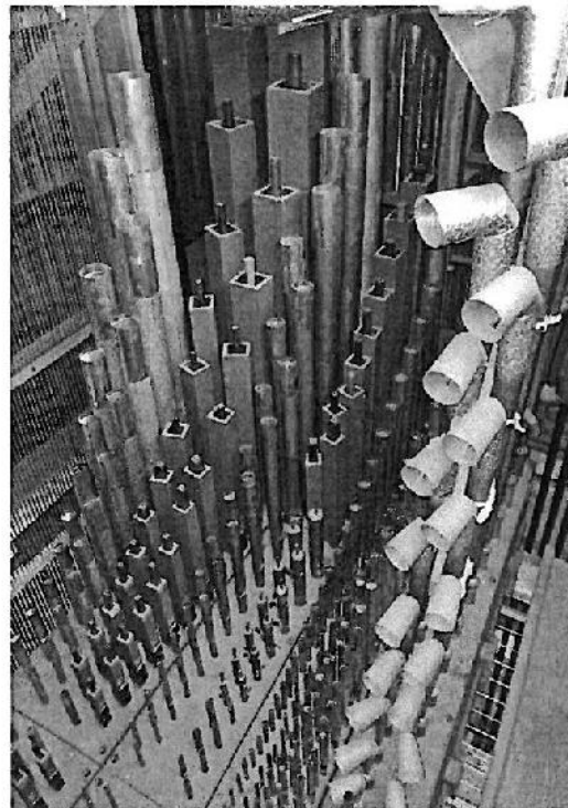
Great pipework showing dust build-up
